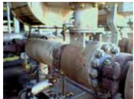
This clamped end CA-HO1 10-inch ASME 2500 class catalyst valve installed in 1995 is still in service at a major Italian refinery.
