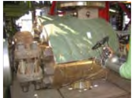
Located in a frigid Scandinavian environment, this large bore ASME 4500 class metal seated ball valve is installed on the outlets of the hydrogen heater.
