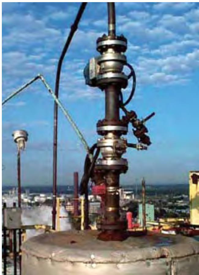
Located at the top of a major refinery, these MOGAS valves were chosen for their performance and low maintenance. Due to their location, reliability was a critical part of the installation decision.
