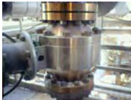
This CA-DRI 8-inch ASME 300 class valve has been handling catalyst at 1425° F / 774° C for numerous years. It is the major isolation valve between the third stage and fourth stage cyclone separator.
