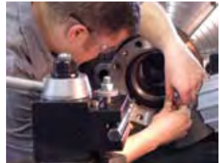
As part of a repair, the MOGAS service technician checks the depth of the seat pocket to certify original design specifications are accurate.
