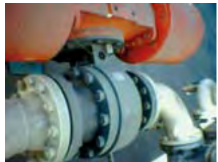
This CA-1AS 6-inch ASME 300 class feed isolation valve is a critical part of the emergency shutdown system.
