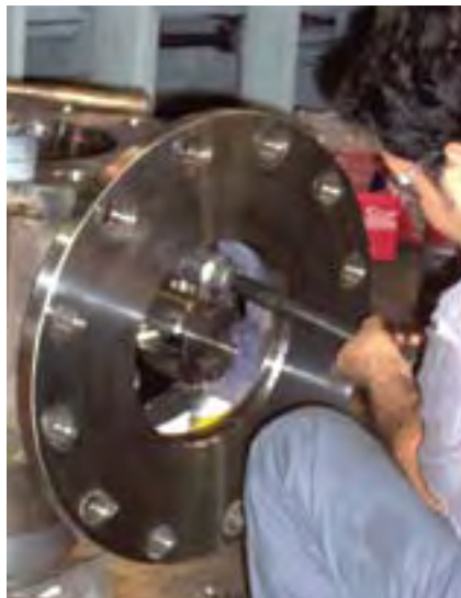
Adjusting the packing gland on a newly repaired valve will ensure the integrity of the energized stem packing.
